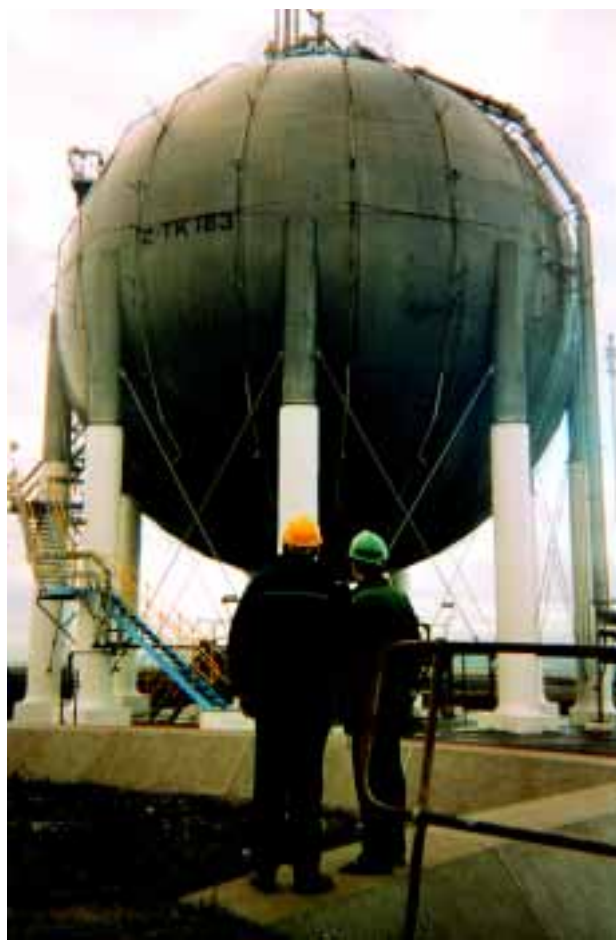
A storage vessel on the 1,000 acre plant at Baglan Bay
