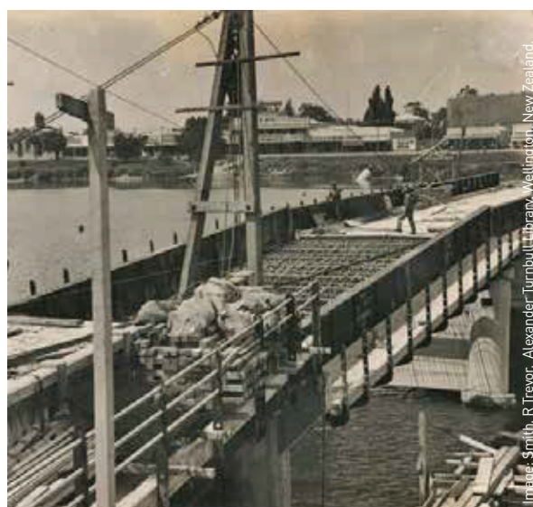
Wairoa River Bridge, Wairoa, Hawke's Bay, under repair after the 1931 Hawke's Bay earthquake.
