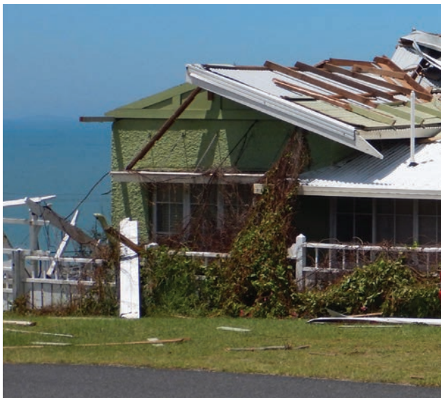
Severe roofing failure due to weak roof framing connections in properties happened during Cyclone Marcia in 2015 in Yeppoon, Queensland. Image: Cyclone Testing Station, James Cook University.
