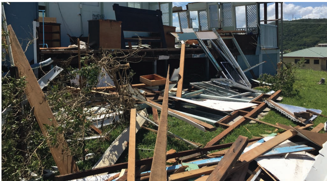
Cyclone Marcia caused significant damage to property in Yeppoon, Queensland due to its severe winds and the way properties were constructed. Image: Cyclone Testing Station, James Cook University.
