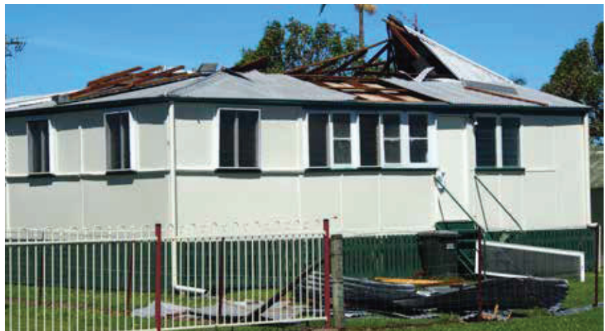
Figure 1: Severe structural roofing failure in Proserpine from Tropical Cyclone Debbie.
